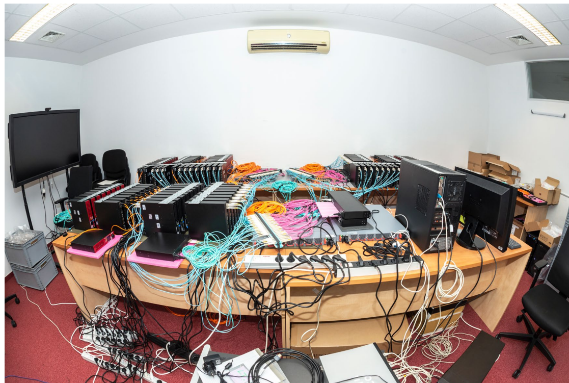
More than a bundle of colorful cables - it's a living video matrix
