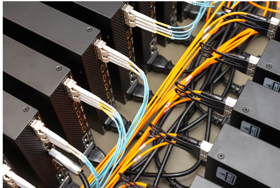
SFP+ transceiver modules, optical cables and SFP+ AOC during the system test
